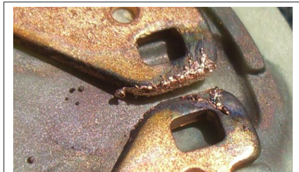
Figure 9 Degraded Gaps of a Station Class Arrester
