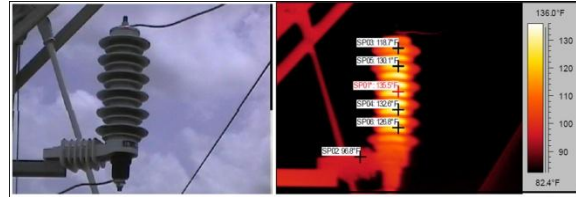
Figure 9 Distribution Arrester with 15C difference between hottest spot and cooler part of the arrester
