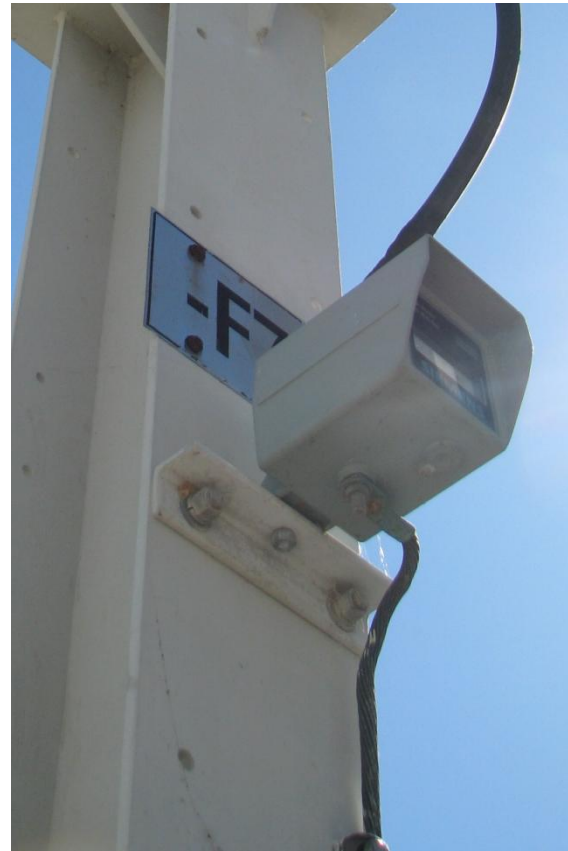
Figure 1 Surge Counter mounted on an arrester pedestal
