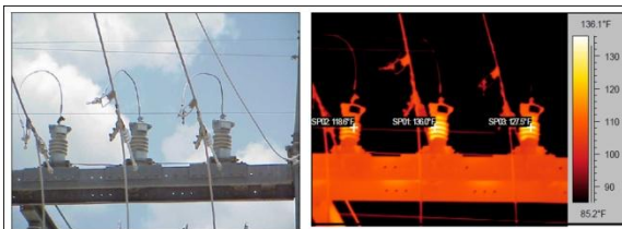
Figure 8 Substation Class Arresters with one unit about 9 C higher than the coolest unit
