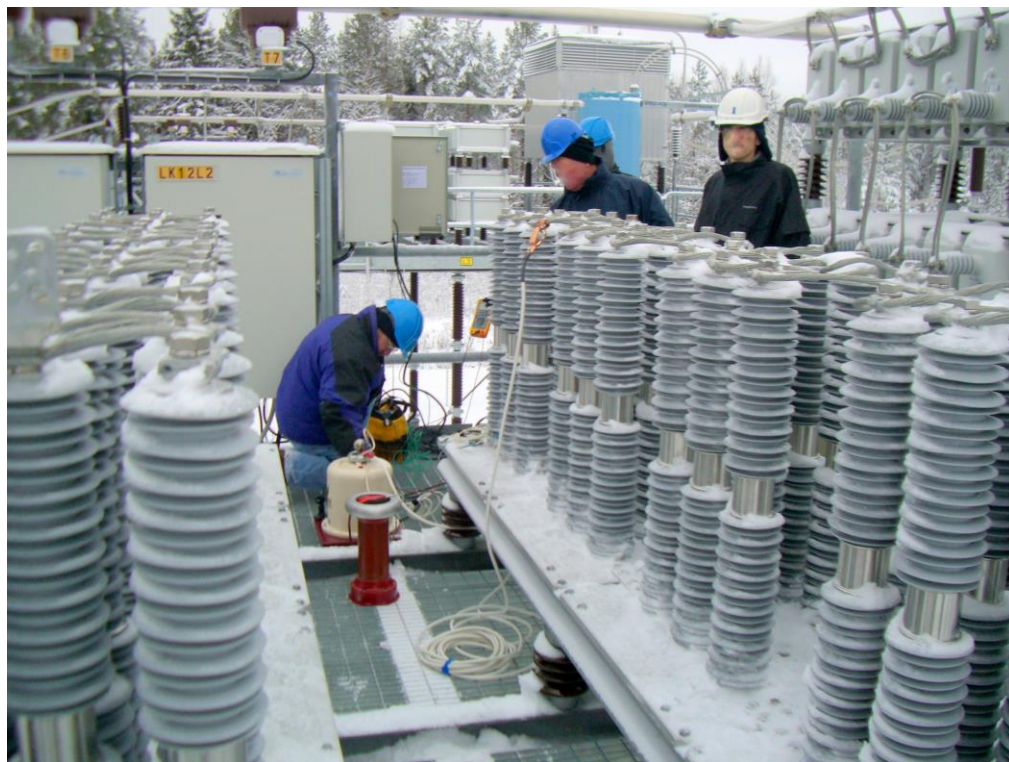
Figure 6: Hipot Testing Varistor Columns in a Series Capacitor Installation
